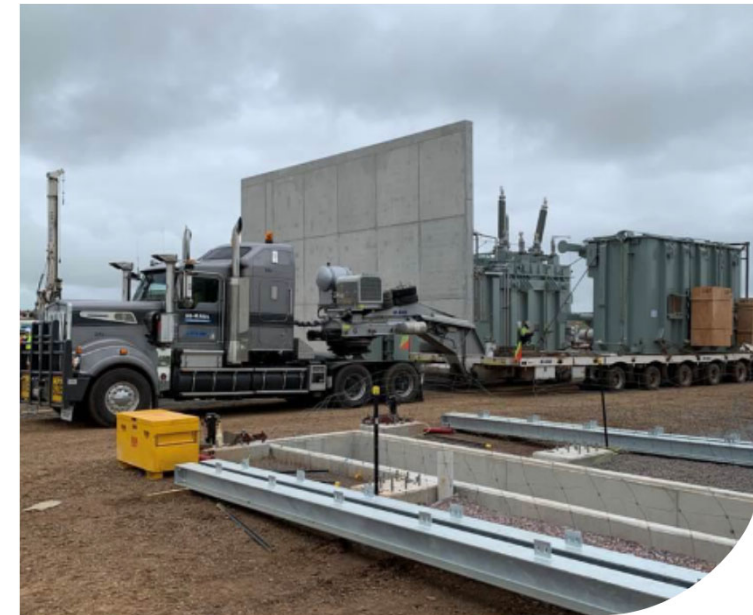
Installed wind farm transformers
